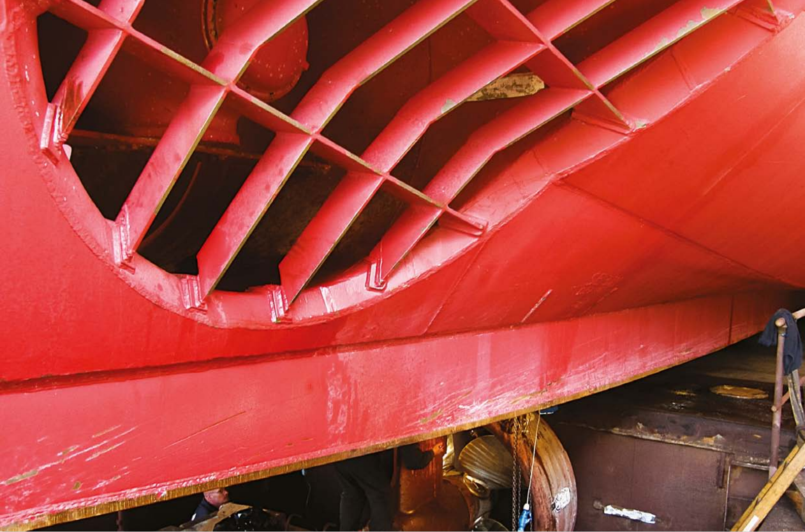
Examples of the minor scrapes and chips which were the totality of the damage to the Ecospeed coated hull after two seasons in the ice.
