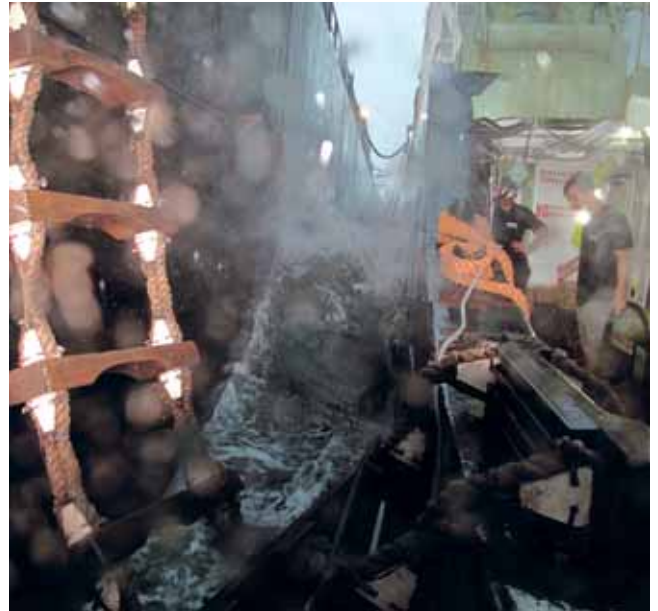
Stormy weather conditions did not stop stern tube seal repair in Manila.
